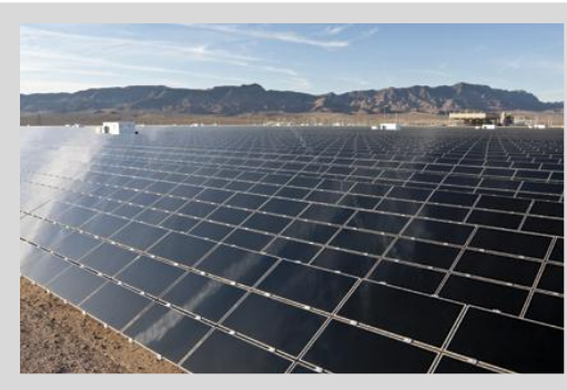
The Copper Mountain Solar Project in Boulder, Nev. is the largest operating PV facility in the U.S.. Already at 58 MW, the facility is scheduled to add an additional 92 MW of capacity by the end of 2012.
