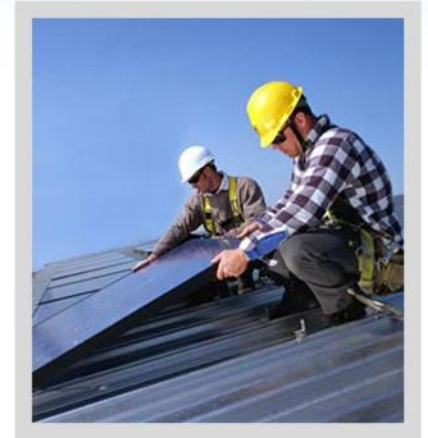
Workers mount PV modules on a private home. These modules use sunlight to generate clean, pollution-free electricity and can reduce or eliminate monthly electricity bills. In 2010, 260 megawatts (MW) of PV were installed on over 48,000 homes.
